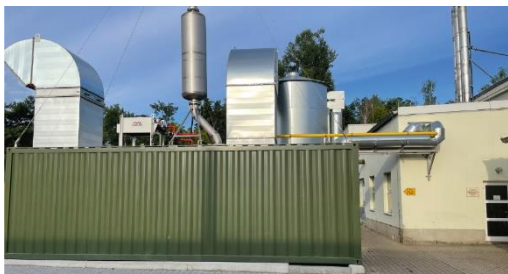
The combined heat and power plant covers an area of 30 m 2 .
