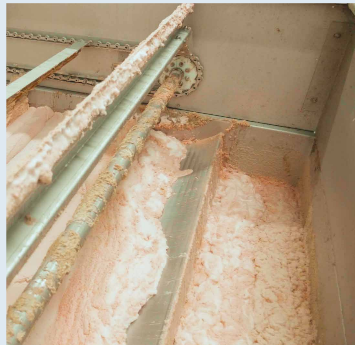
The Aeco-Fat plant at Esbro, which generates valuable resources through fat recovery, has been in operation since 2019.
