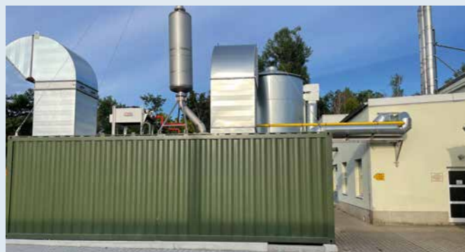
CHP unit covers a total area of 30 m 2 .
