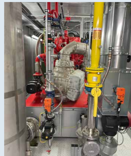
The heart of the plant is an 8 cylinder gas motor with a generator.
